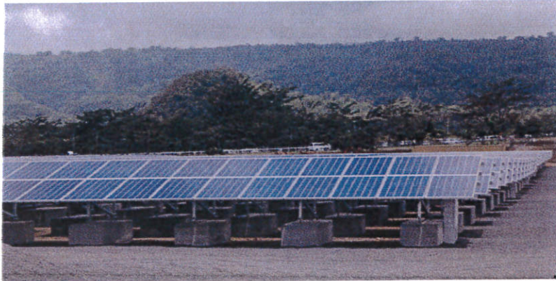
The Apia Racecourse Solar Array. Photo / Henrietta McNeill
